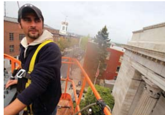
Dana Martin of Grime Solutions of Carlisle, gets a birdseye view of the Adams County Library in Gettysburg while working to clean the historic structure. GETTYSBURG TIMES PHOTO
